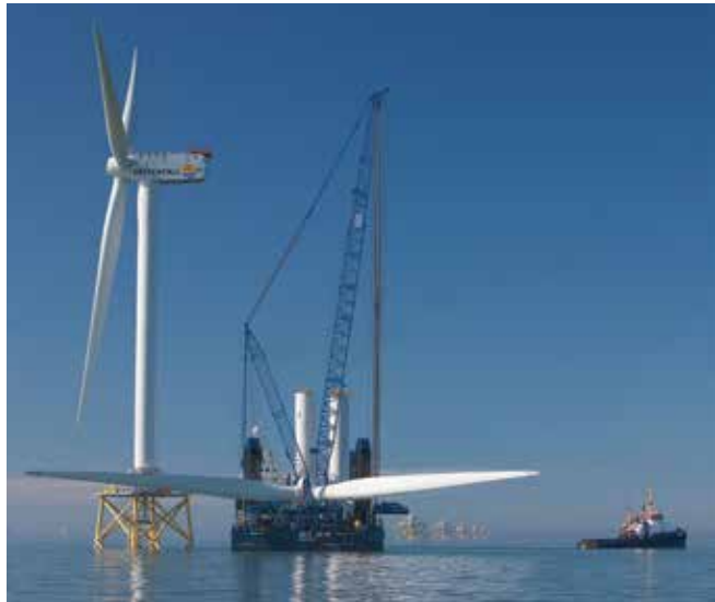
Jacket foundation at Ormonde
